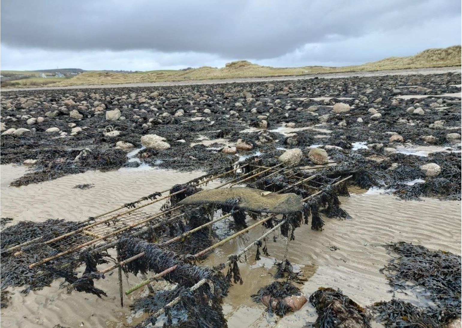
Figure A4.4 Remnants of abandoned trestle on the foreshore at Warren Beach
